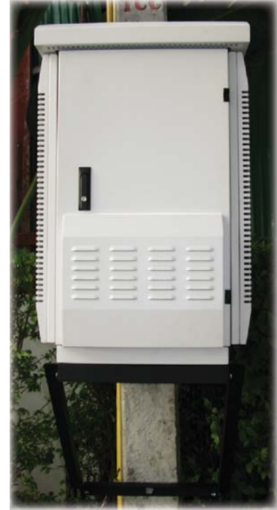
Cabinet on Pole
